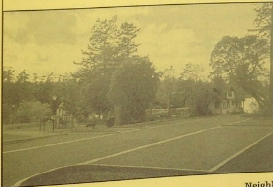
Construction of the new parking area at Gorge Waterway Park and the Victoria Canoe and Kayak Club is well underway.
